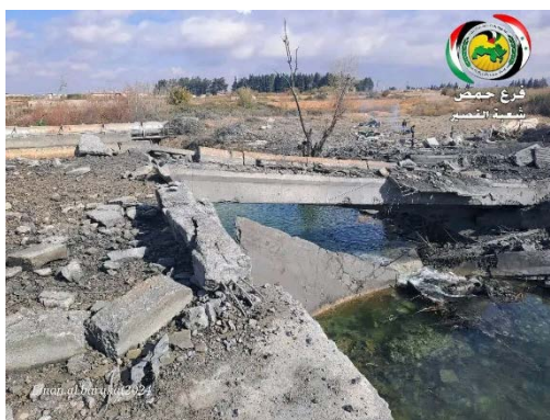
A bridge destroyed in an IDF attack (SAM SYRIA Telegram channel, November 26, 2024)
