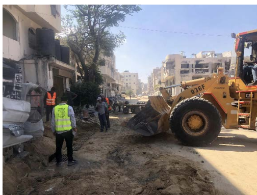
Repairing the drains in Khan Yunis (Khan Yunis municipality Facebook page, September 29, 2024)
