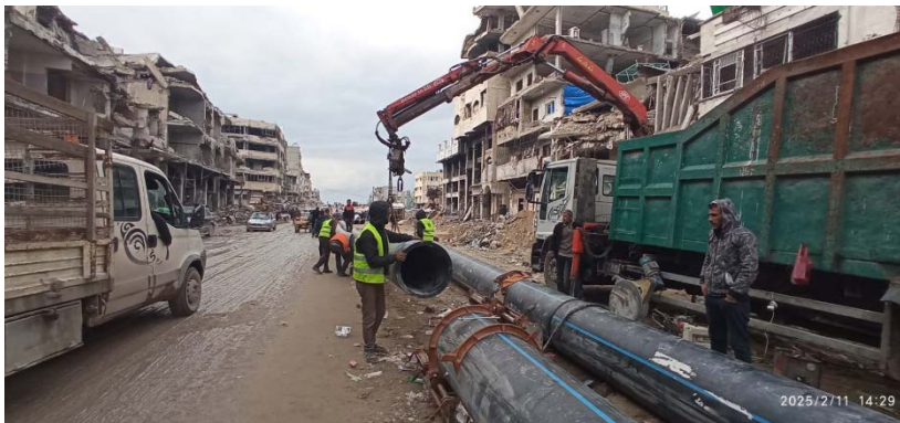
PA water commission workers install pipes in the Gaza Strip (PA water commission Facebook page, February 12, 2025)
