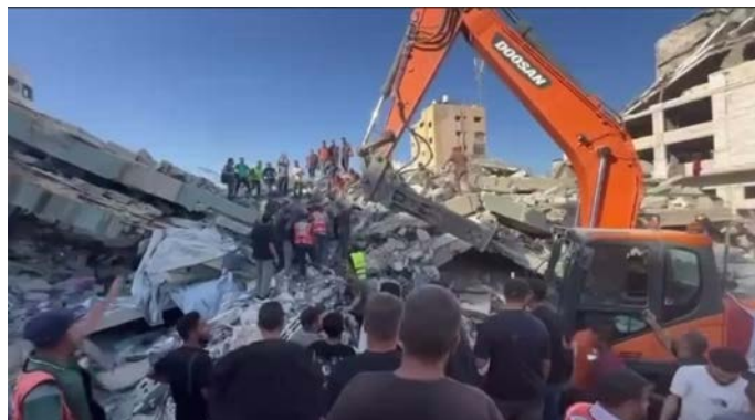
Rescue operations at the collapsed building (Shehab Agency, September 16, 2026)
